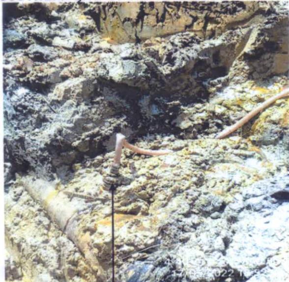
SPILL POINT (1"galvanize pipe with hose connected to the 3" valve at 12 O'clock position on the 14" pipeline)
